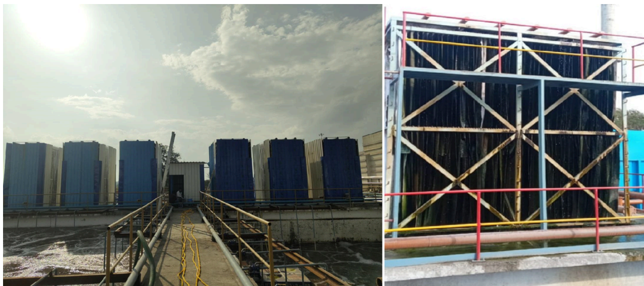
Figure 4. Field-scale installation of the Algal-Bacterial Attached Growth System, commissioned at a sugar-distillery effluent treatment plant.
